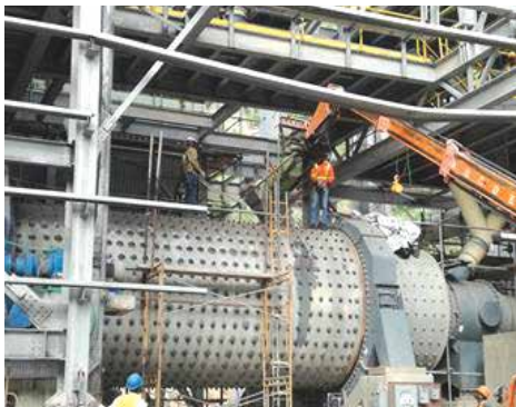
New Coal Grinding System at CCCL
