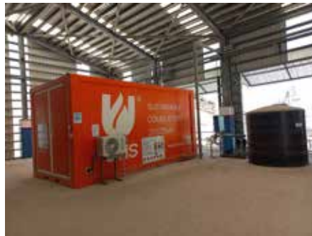
JAM: Transformer and UTI's
