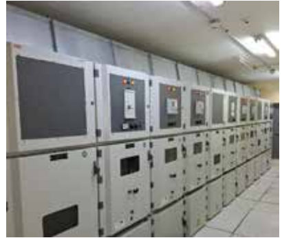
JAM: Breaker for new Transformer
